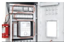
Electrical Cabinets Suppression
